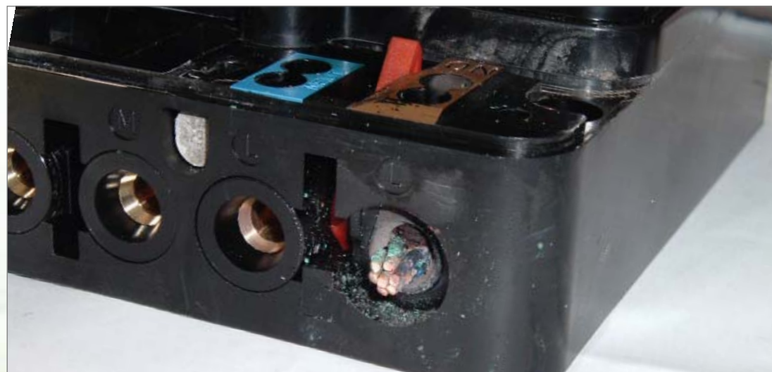
BURNED CONNECTION ON CONTRACTORS SIDE OF METER
